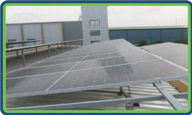
275Kwp Rooftop Solar System Installation & Commissioning At S.R.METALLIZERS, Hoziwala Industrial Estate, Sachin, Surat
