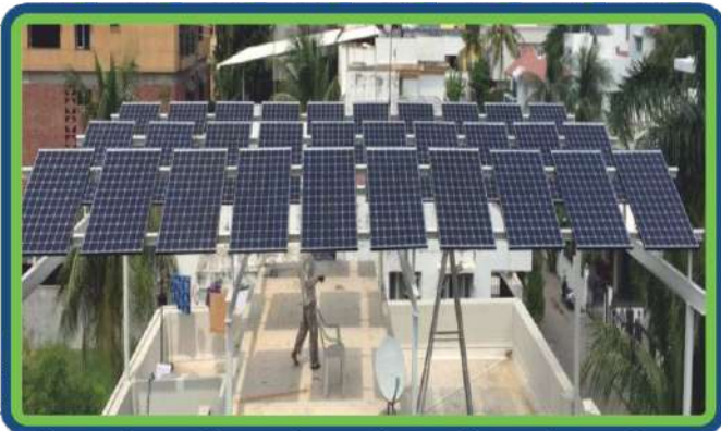
10 Kwp Rooftop Solar Mr. Vijay Kaniya, Athvalines, Surat.
